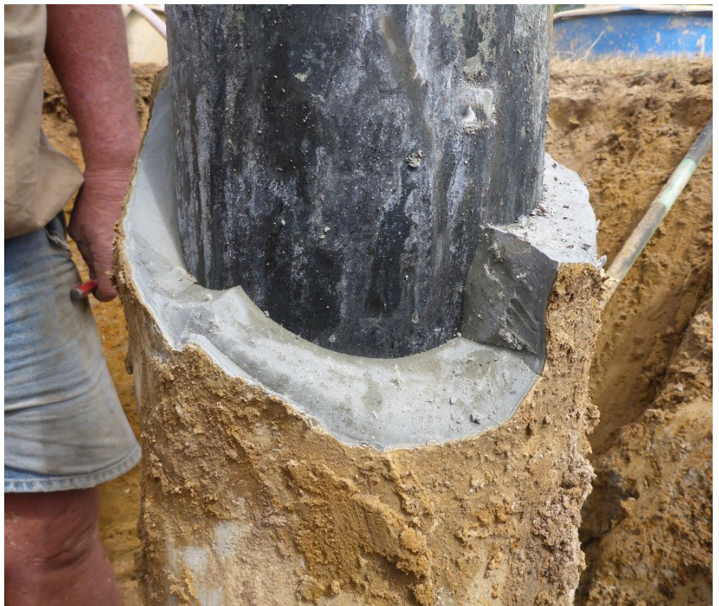
Casing centred in the bore hole with uniform grout seal around the casing
